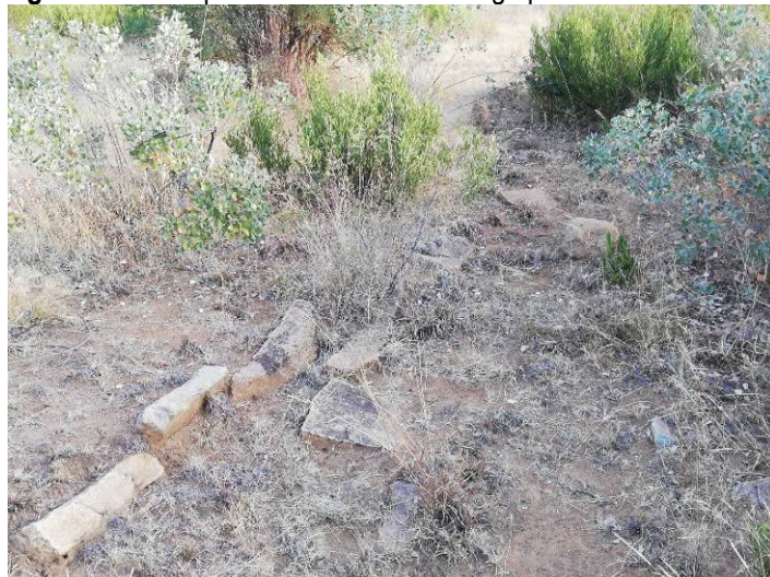
Figure 11: Example of dilapidated linear walling.
